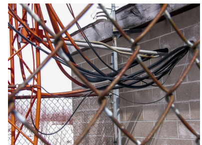
tangle of cables
