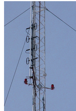
lights, more antennas at 150'
