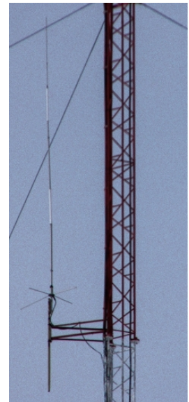
repeater antenna, base at 80'
